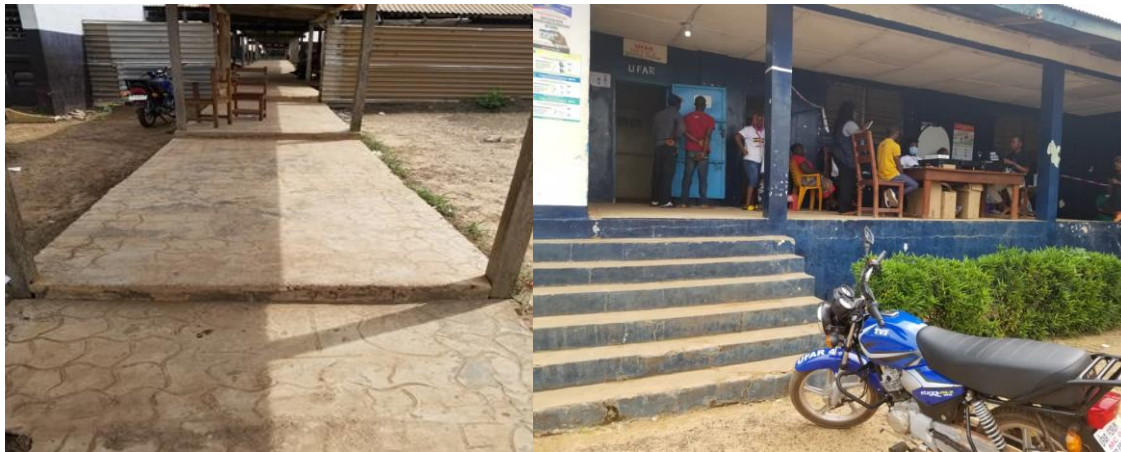
Figure 2: Two registration centers in Grand Gedeh County located at LOIC Youth Building and Zwedru Multilateral High School where access for persons with disabilities is limited due to stairs.
